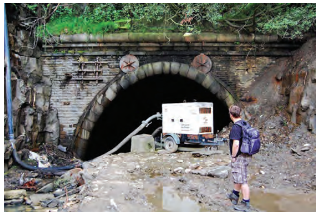
The south portal of Queensbury tunnel in 2012 after the water had been pumped out of the Strines cutting to allow maintenance of the tunnel.
